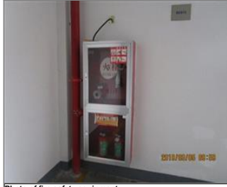
Photo of fire safety equipment Fire hydrant and fire extinguishers.JPG
