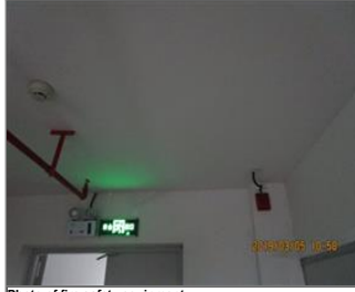
Photo of fire safety equipment Fire alarm.JPG
